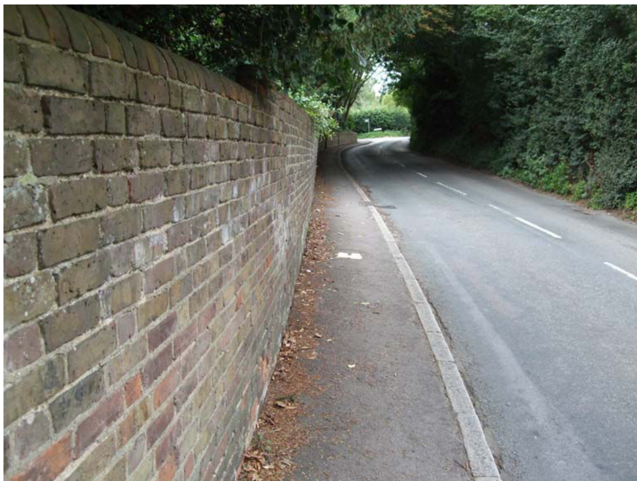
Boundary Road Wall requiring to be stabilised or or rebuild 15M Length
