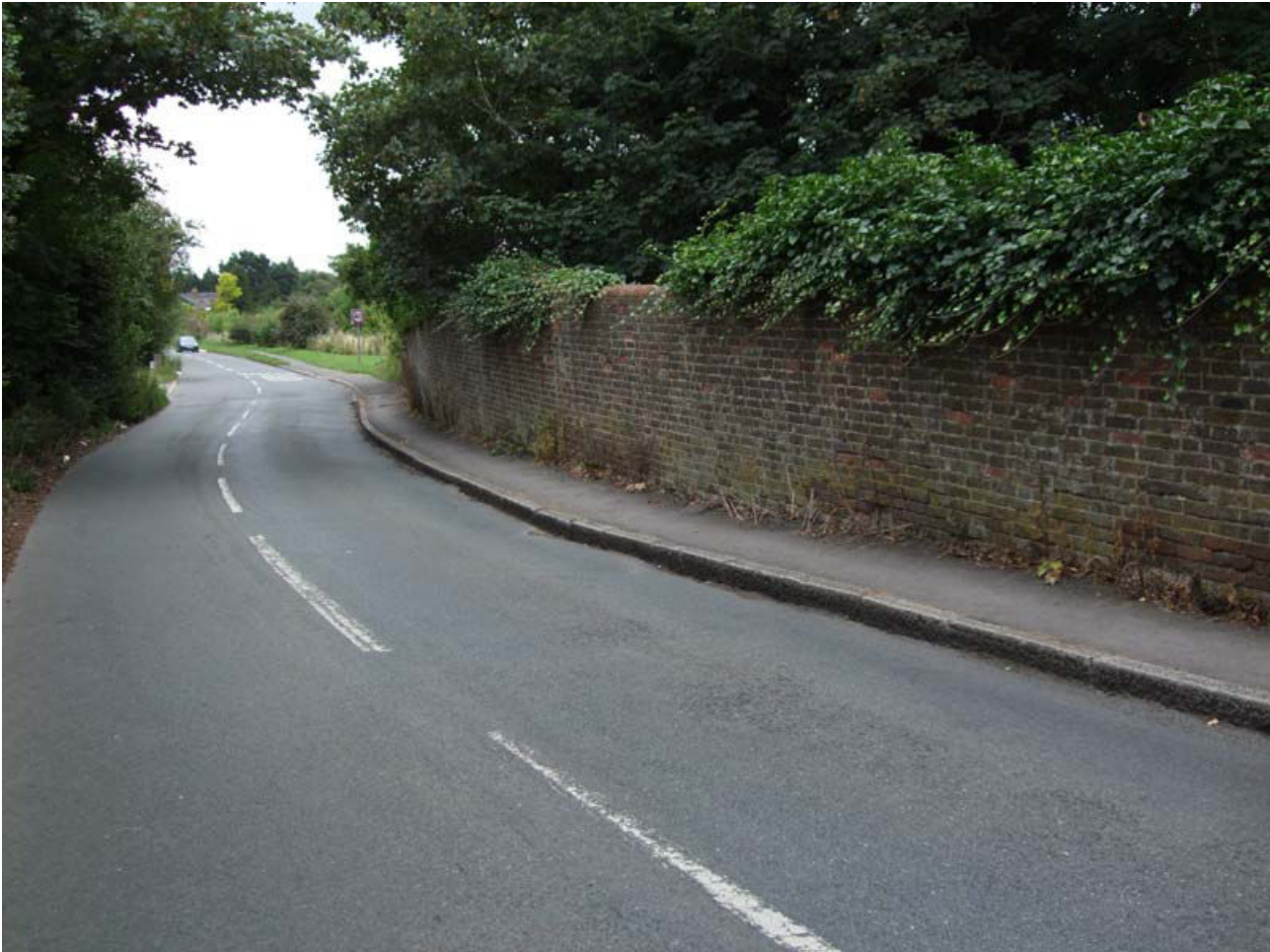
Boundary Road Wall requiring to be stabilised or rebuild 15M Length
